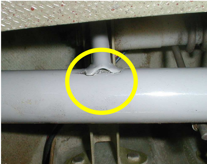
picture 3: Damage viewed from front
